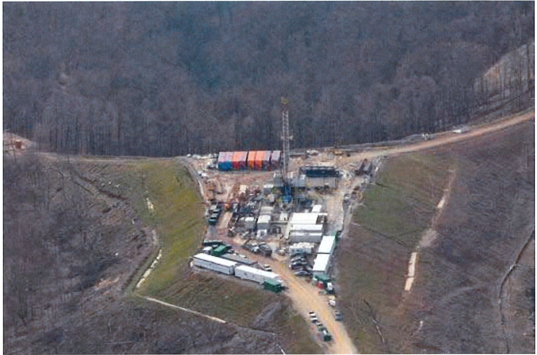
Fracking imposes a range of environmental, health and community impacts. Above, a fracking well site is built in a forested area of Wetzel County, W.Va. Credit: Robert Donnan
